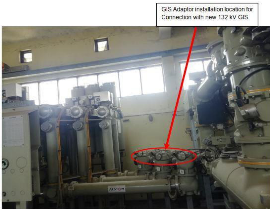
Figure 1 : GIS Adaptor at Existing 132 kV GIS
