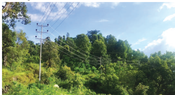
Newly Constructed Malekhu-Dhadingbesi double circuit 33 kV subtransmission line
