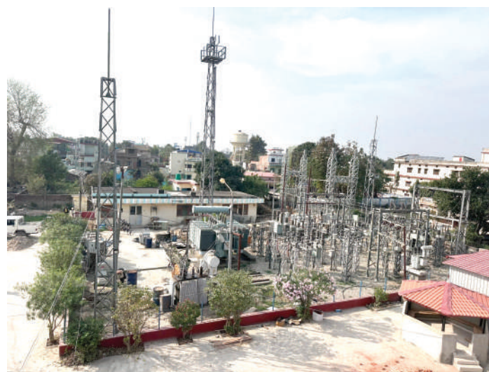
Gulariya Substation with SAS and VMS facilities
