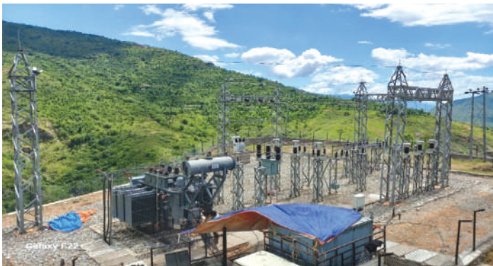
33/11 kV, 6/8 MVA Tumbewa, Panchthar Substation Completed.
