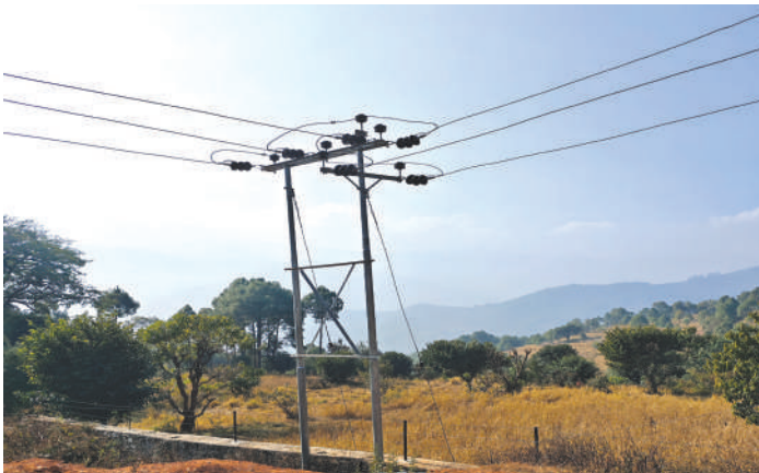
33kV line structure at Namdu substation
