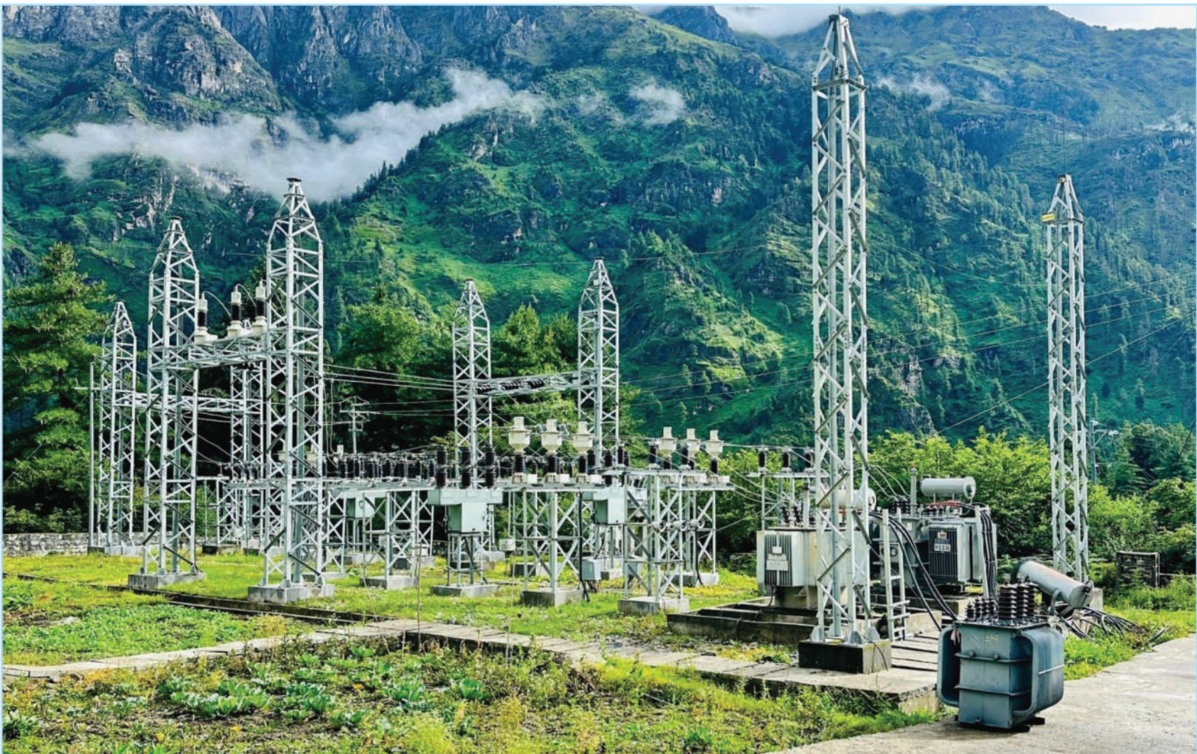
Sharkhu Substation Manang
