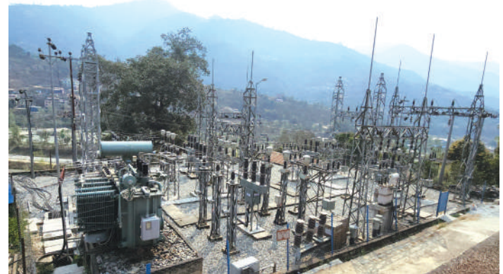
33/11 kV, 8 MVA Manthali substation, Ramechhap
