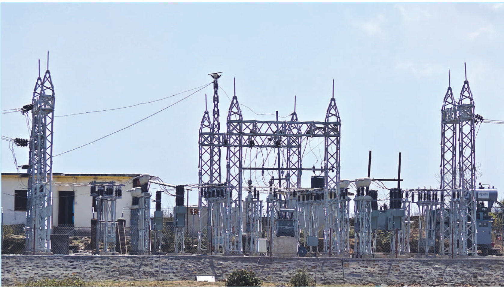
33/11 kV, 8 MVA Tute substation, Tehrathum
