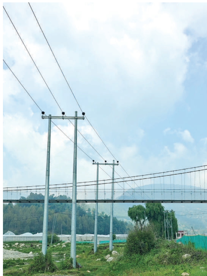
33 kV H pole-structure for crossing of suspension bridge at Palung
