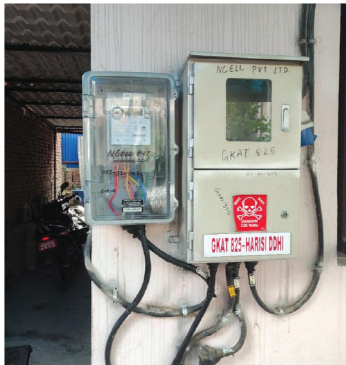
Smart 3 Phase Energy meter installed at consumer site
