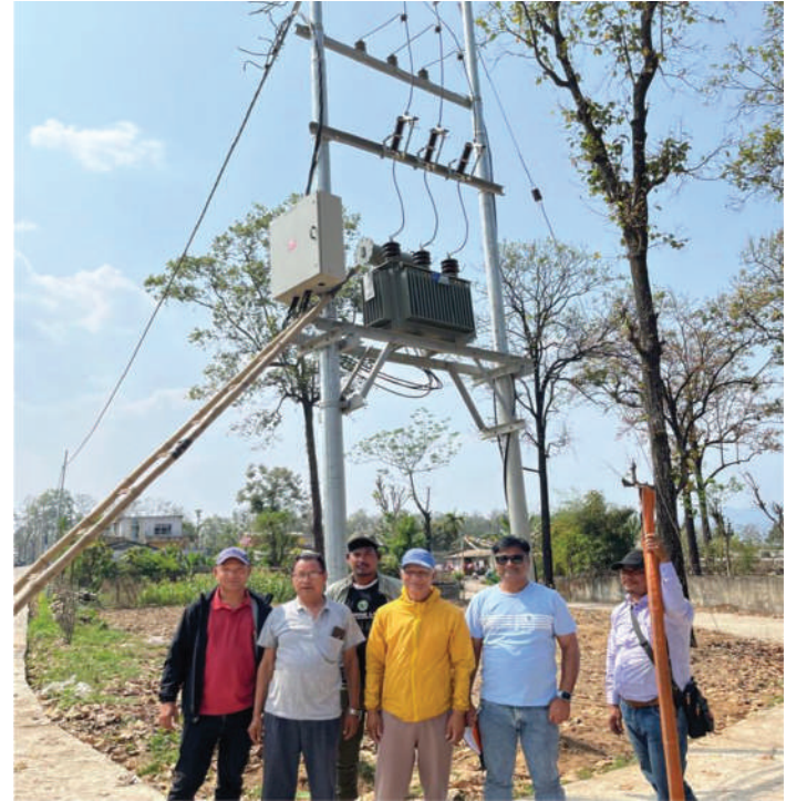
A Distribution Transformer successfully charged at Makwanpur site
