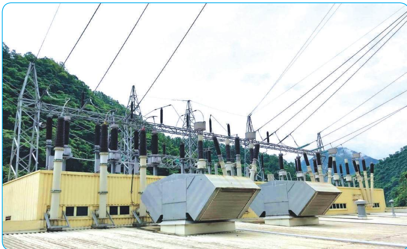
Switchyard of Marsyangdi HPS
