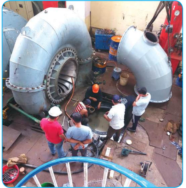
Dismantled view of spiral casing
