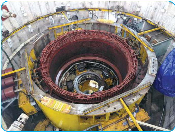
Stator of unit 2
