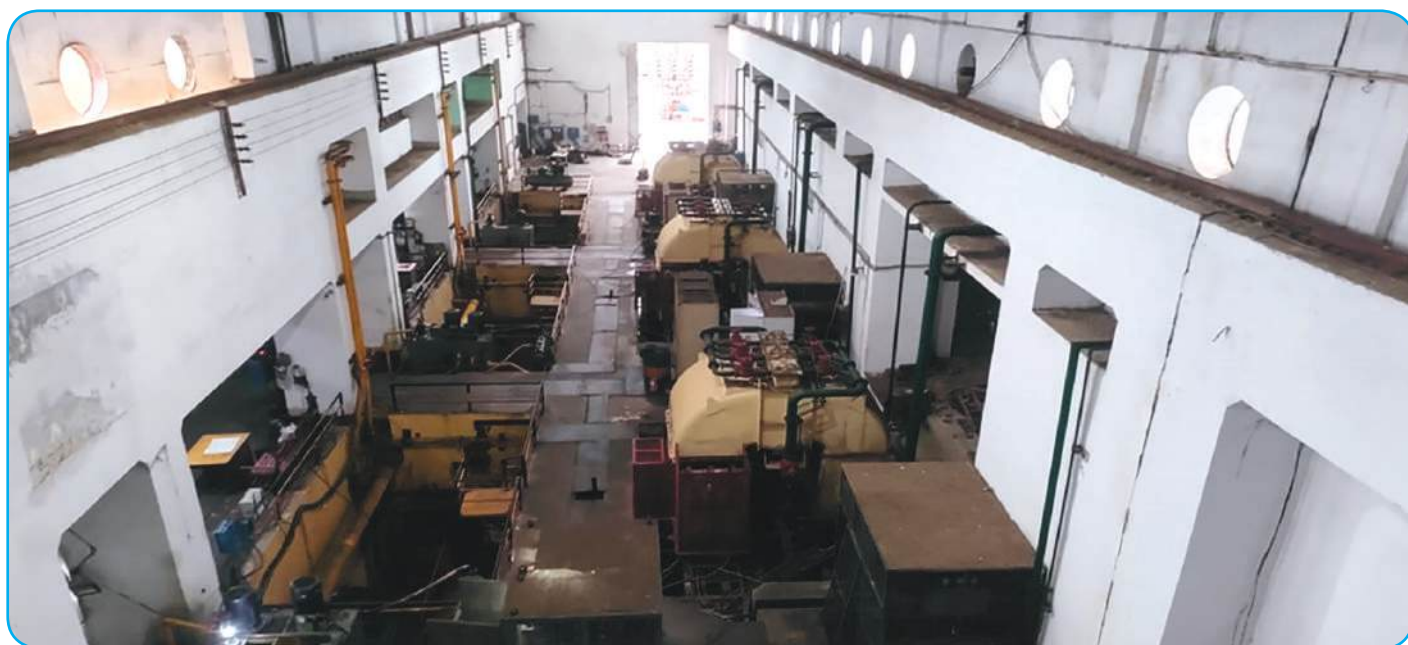
Unit bay of Gandak HPS
