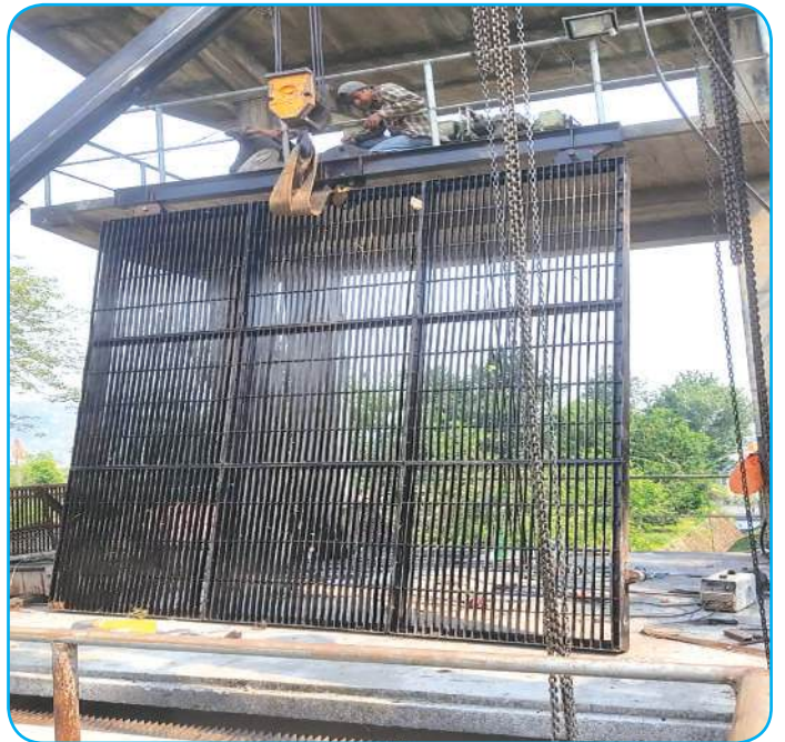
Trash rack with hoisting
