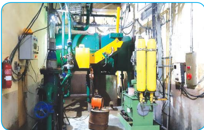
View of MIV from the turbine floor
