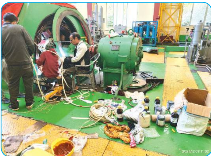
Repairing of 3700kVA synchronous generator stator coil of unit#02 with new terminal cable
