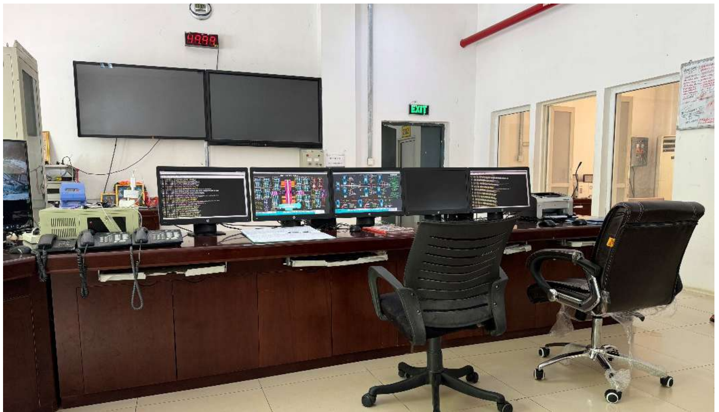
Control Room of Upper Trishuli 3 'A'
