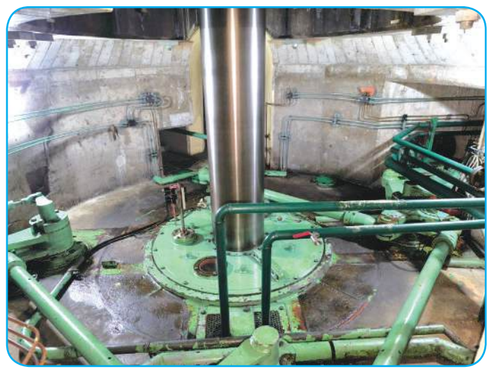
View of turbine shaft and link rods
