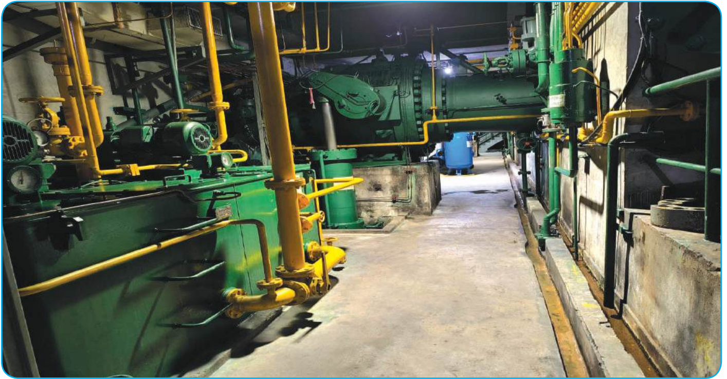
View of MIV and Oil reservoir tank
