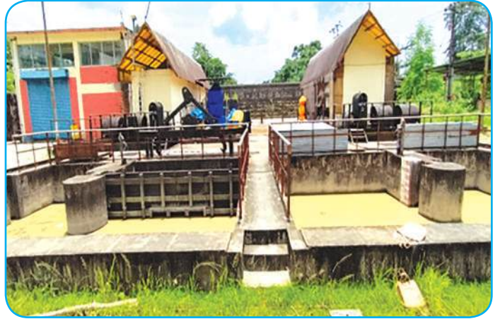
Chatara HPS with Intake and Gates
