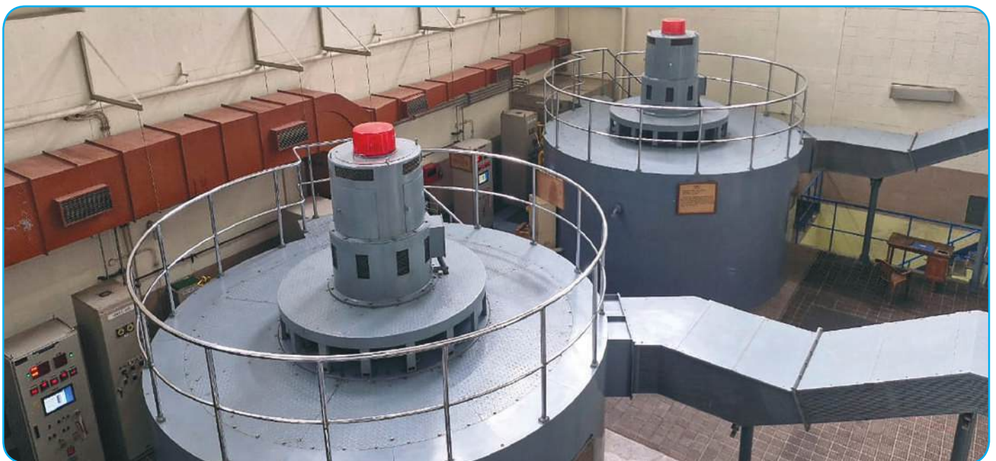
Generator floor of Kulekhani II HPS
