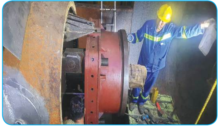
Piston Cylinder Assembly Works for Unit 3
