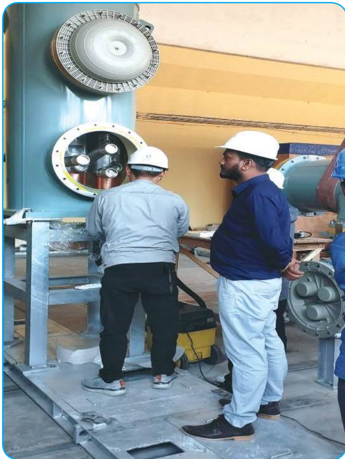
Extension of two GIS bays
